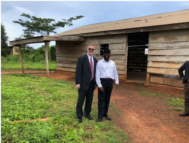
This was taken outside the church last October. As you can see the building was in extremely poor condition
