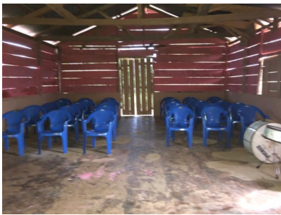
THE CONCRETE FLOOR IN PLACE OF THE DIRT ONE AND THE NEW PLASTIC CHAIRS HAVE BROUGHT GREAT EXCITEMENT TO THE CHURCH
